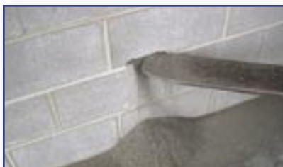
Loose fill drains out of the wall if puncture occurs, with no way to reinstall it.
