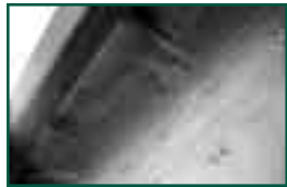
Figure 5: Note the tight seal developed around the roof trusses and the roof-wall juncture.
