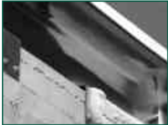
Figure 4: SPF application at the roof-wall juncture. The spray pattern can be seen at the lower right corner of this photo.
